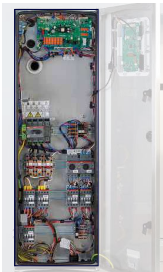
Single-point power connection
