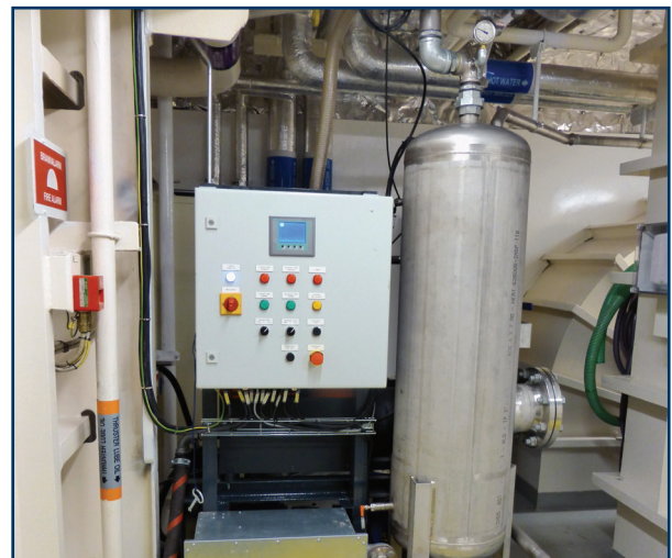
On board installation of Vacuum unit VU-65.
