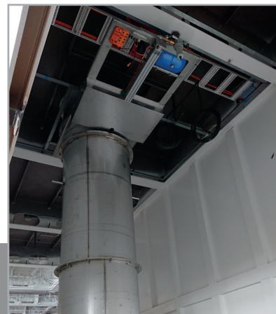
Fig. 3: Fire shut-off guillotine
